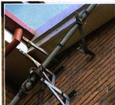
You can't defy the laws of gravity: These two wall brackets are too close together, putting tremendous strain on the whole setup
